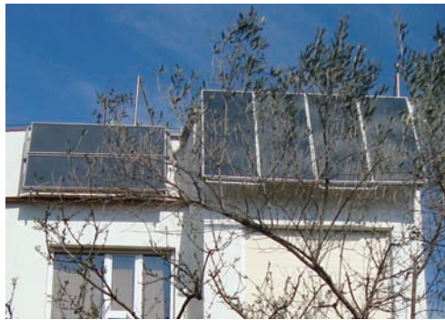
Figure 2. Solar panels to provide hot water and heating
